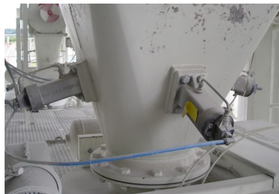
multiple PKL 740 with self-control (ST-Kit) mounted on cement powder hoppers
