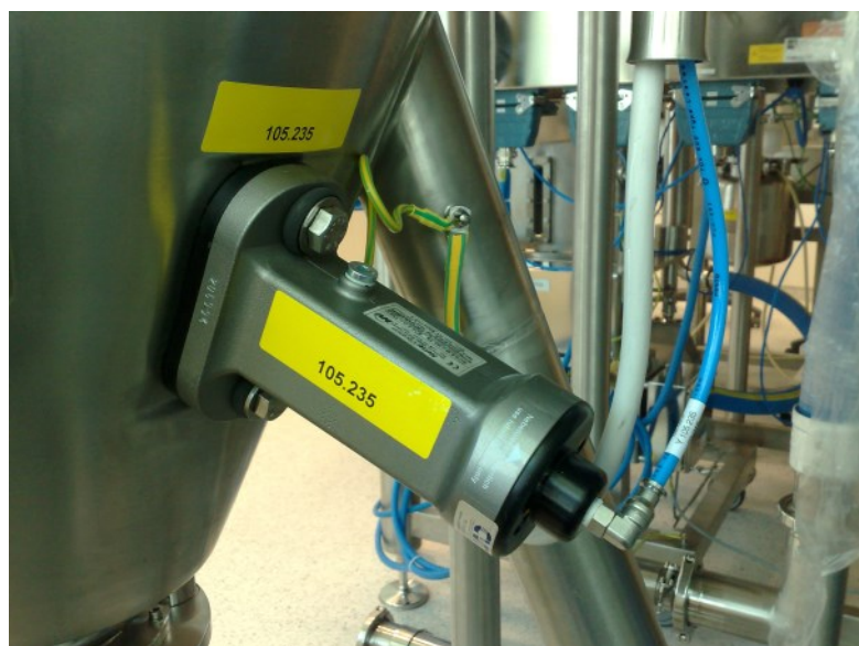
PKL 450 ATEX installed in pharmaceutical industry
