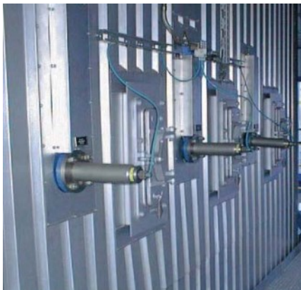
PKL 240 HT is mounted on a large filter, at a power plant
