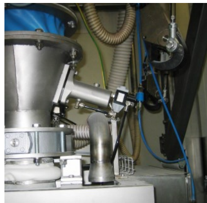
PKL 190 with self-control (ST Kit) mounted on a metering station for powdered materials
